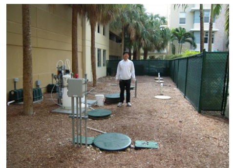
Guanghui Wang with underground collection tanks
