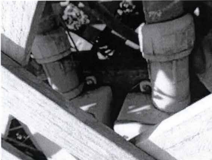
Exemplar of older conduit feeding berth nr 8 and up that was not renewed
