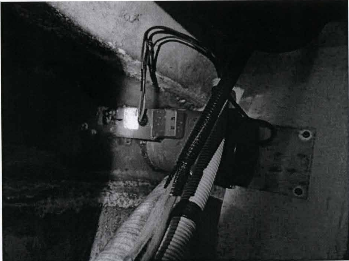
Fwd bilge pump properly wired
