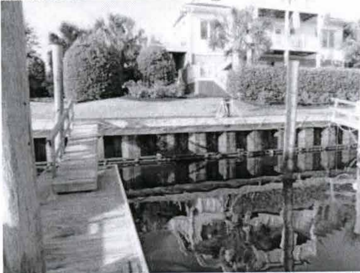
View of nr 7 berth with a rising tide. Note the bulkhead with exposed reinforcement which extends outward approximately 12" from the face. Potential area where swim platform can be caught if boat is not properly secured
