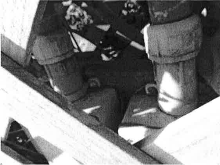
Exemplar of older conduit feeding berth nr 8 and up that was not renewed
