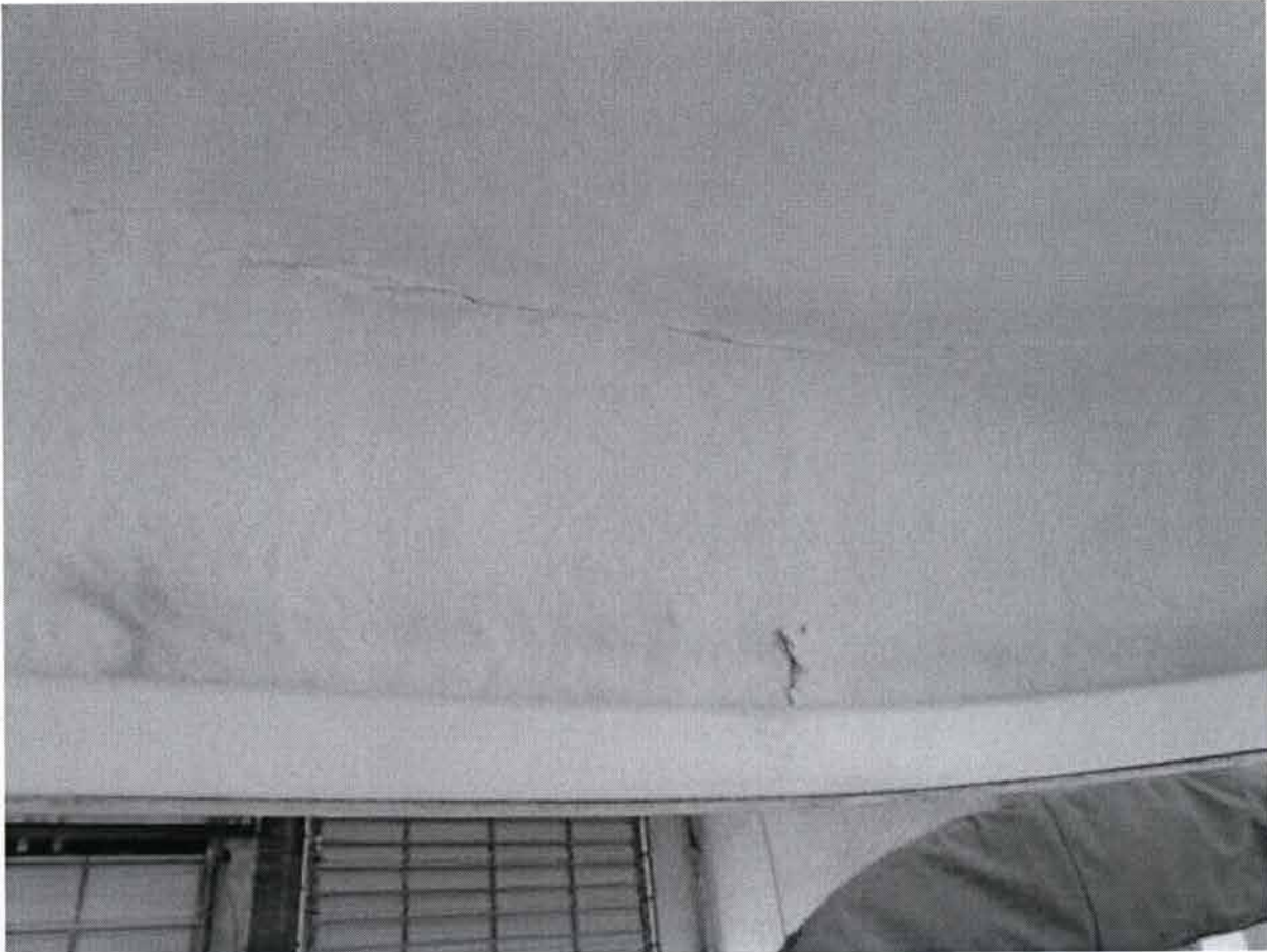
fresh crack in the port side underneath
