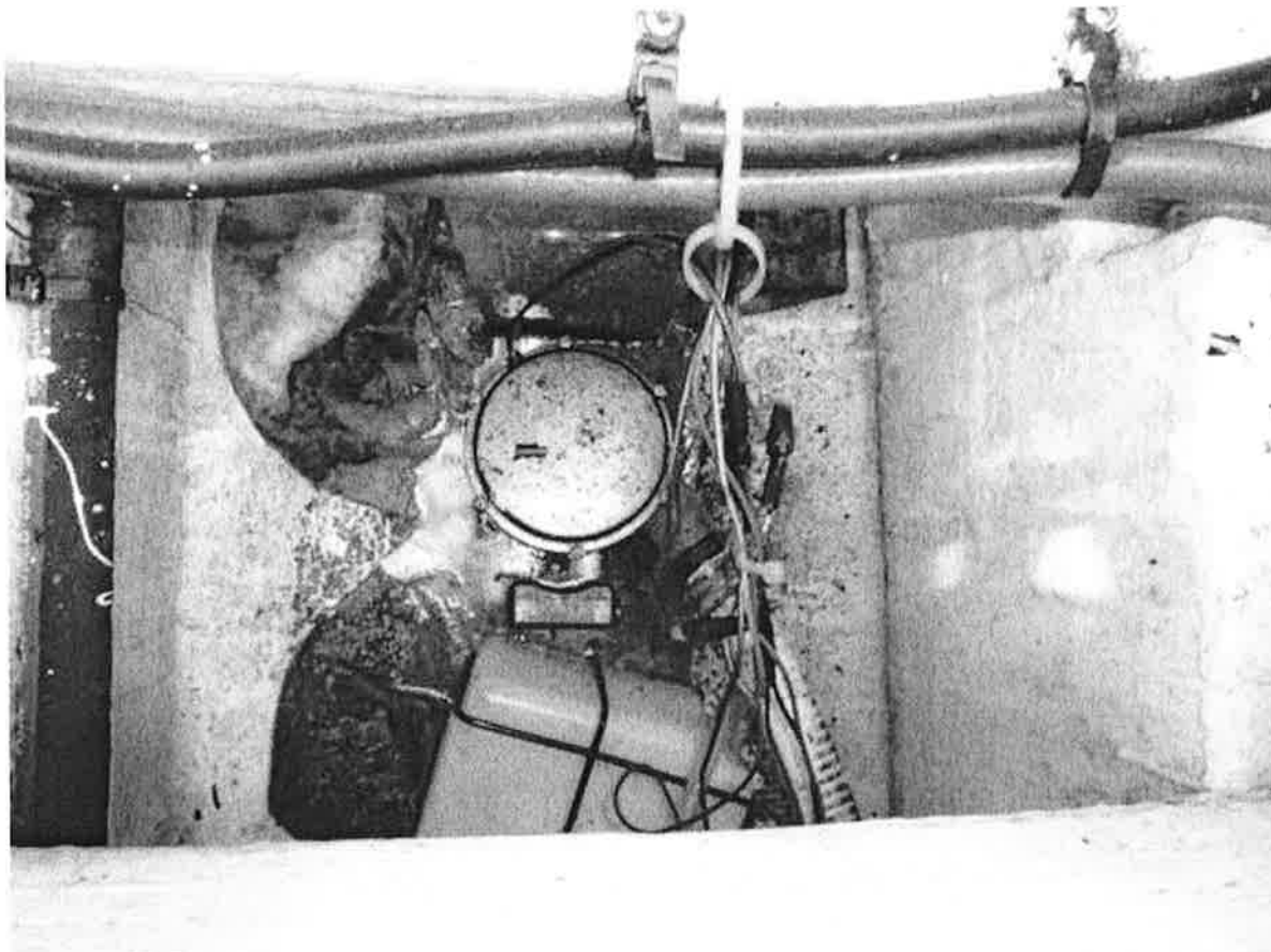
Johnson pump and float switch found properly wired
