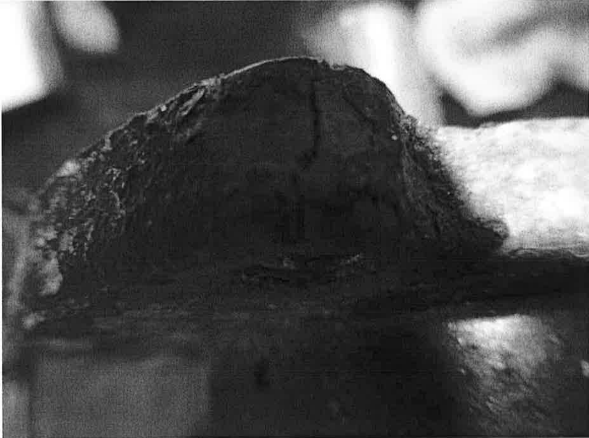
One of cracks where the bolts secure the plastic housing to the pump drive
