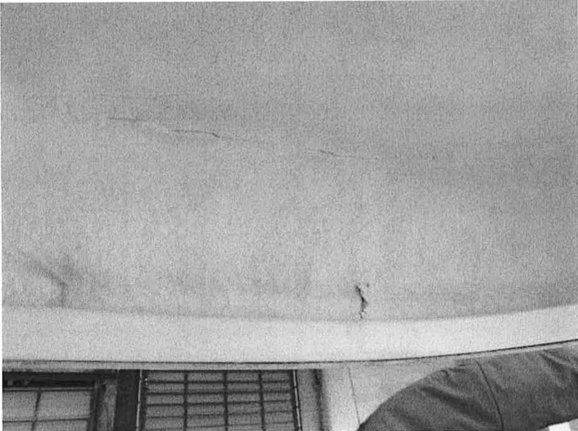
fresh crack in the port side underneath
